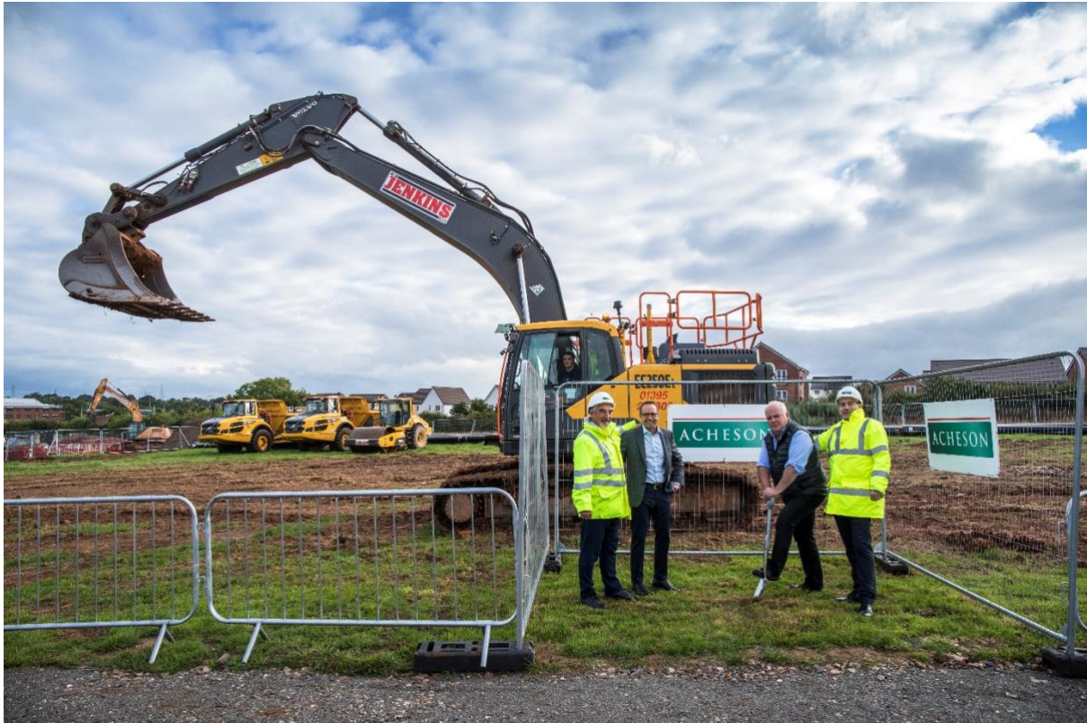
East Devon District Council Leader Cllr Paul Arnott breaking ground alongside (left to right) Acheson Operations Director Colin Johnson, HDDL Managing Director Scott Davidson and Acheson Commercial Manager David Green.
